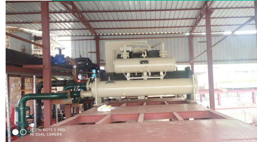
Vapor compression screw chillers with VFD
