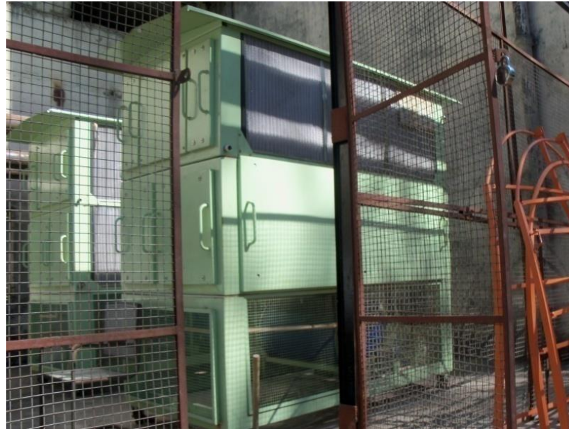
Liquid desiccant dehumidification system
