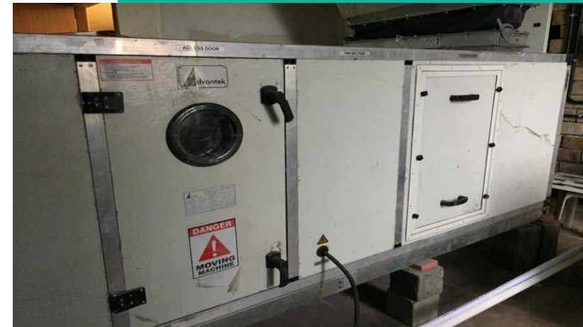
Treated fresh air system with dual coil
