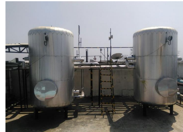
Associated storage tanks for hot and chilled water
