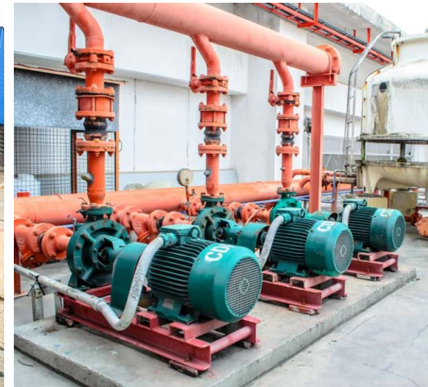
Condenser water pump
