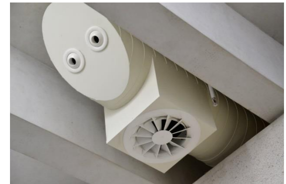
Centralized AC system
