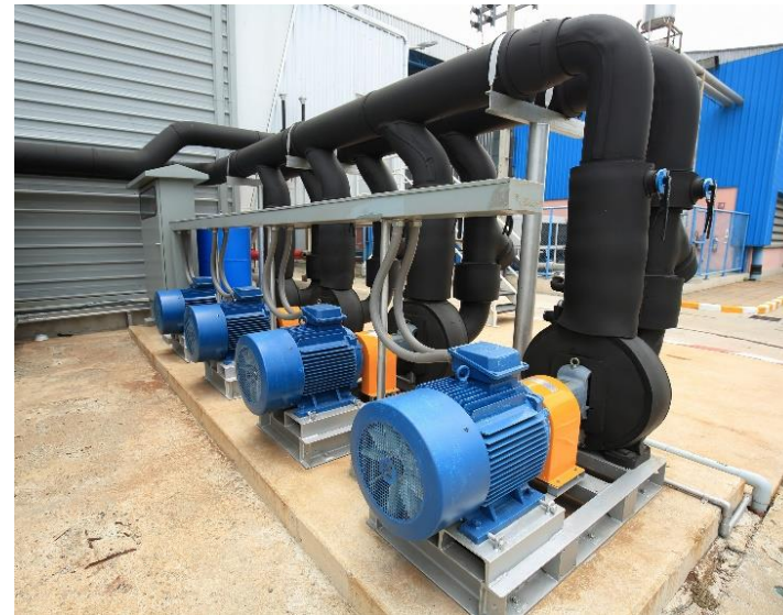
Chiller water pump
